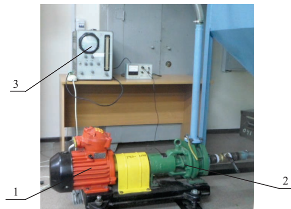
Fig. 11. Installation measuring system: 1 – electric motor, 2 – pump, 3 – vibrometer
